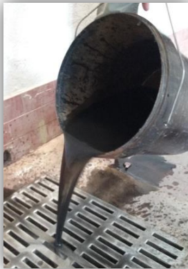
Magnetic filter draining
